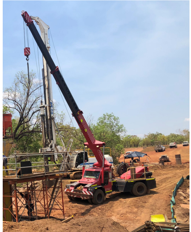
KAMBOLGIE CREEK BRIDGE, NT BY ADVANCE CIVIL ENGINEERING, WINNER OF THE 2021 NATIONAL CIVIL/INFRASTRUCTURE AWARD – UNDER $25 MILLION
