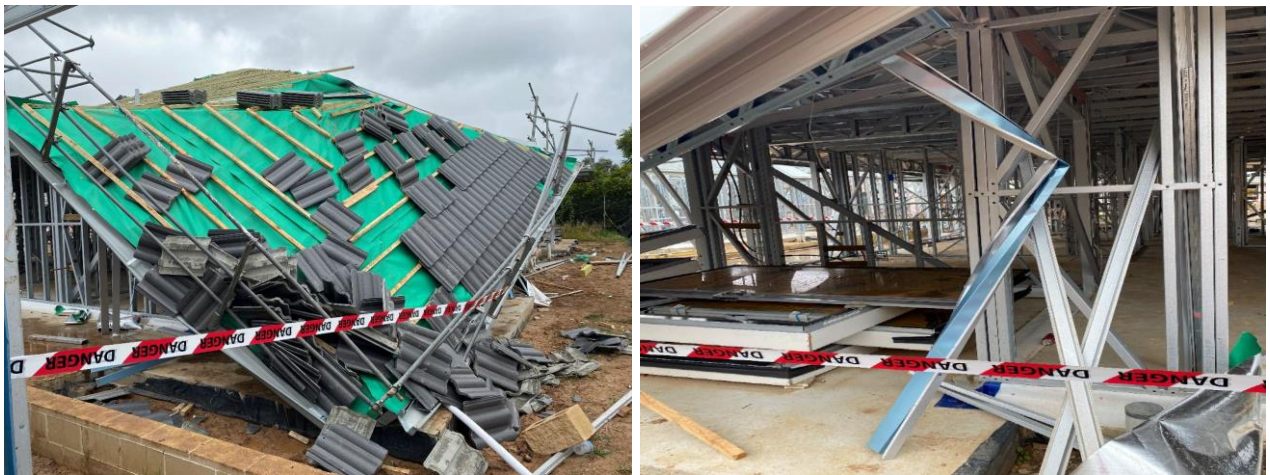
The collapsed roof and the temporary support that gave way.
