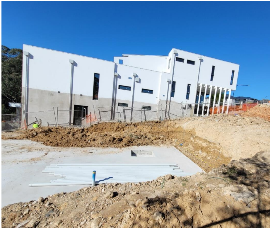
Construction site where the excavation collapse occurred.
