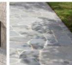
Large pavers or stones bring a contemporary twist to a formal path.
